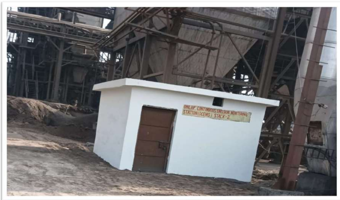
Continuous Emission Monitoring System (Stack 1 & Stack 2)
