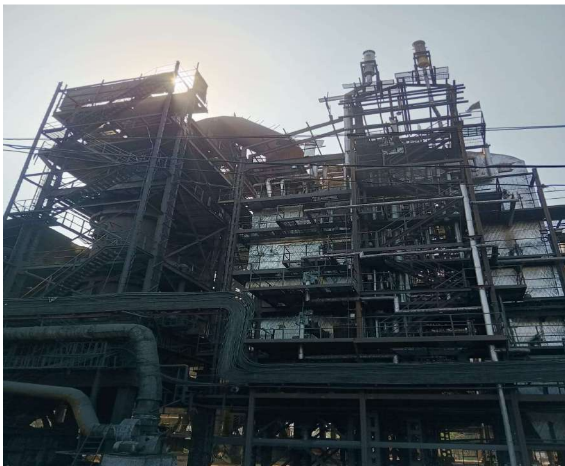
Waste Heat Recovery Boiler (WHRB)
